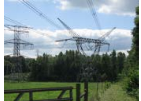
ComEd Transmission Lines
