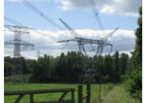
ComEd Transmission Lines
